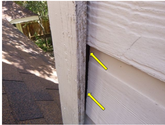
Vertical siding board cut too short.
