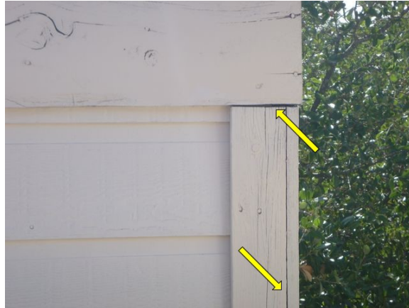
Chimney trim boards are beginning to show signs rot.
