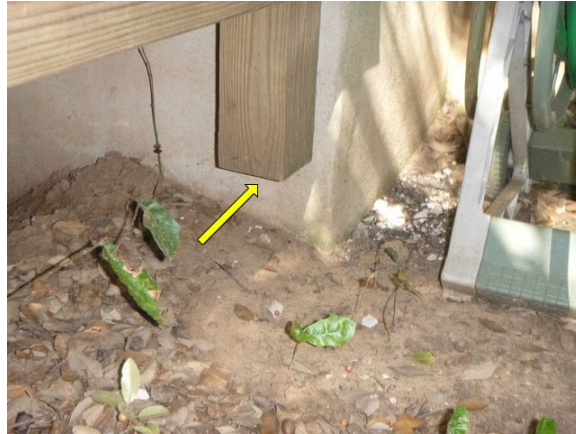
Unsupported piers near house.
