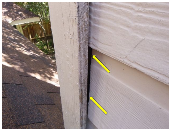
Vertical siding board cut too short.
