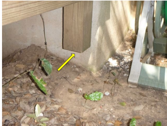
Unsupported piers near house.
